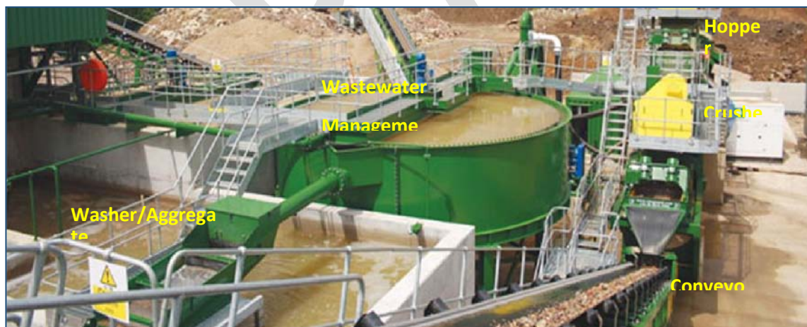
Figure 1.3 - C&D Waste recycling plant in Delhi iv
